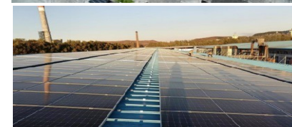
Muling Distributed Power Station ▪ Mudanjiang, Heilongjiang ▪ 799KW
