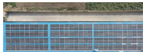
Jiangling Miye Distributed Power Station ▪ Jingzhou, Hubei ▪ 1000KW
