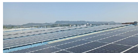
Huaihua Distributed Power Station ▪ Huaihua, Hunan ▪ 1164KW
